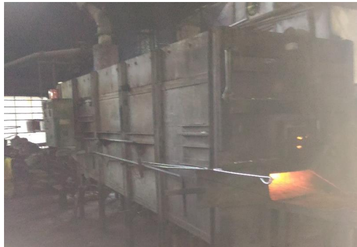
Figure 5: Typical Reheating furnace
